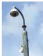
TRAFFIC CONTROL, LIGHTS & CAMERAS
